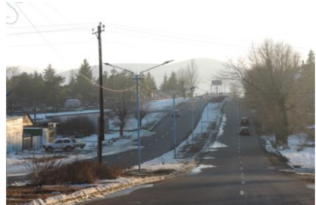
Picture 32: New 75W LED street lights
