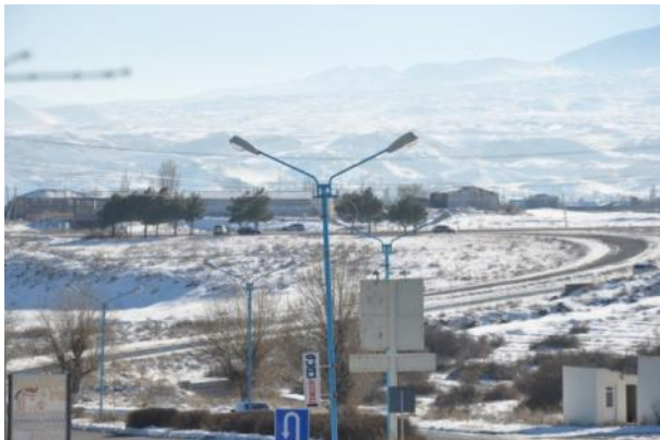
Picture 31: Old luminaries with 250W HPS and MV lamps
