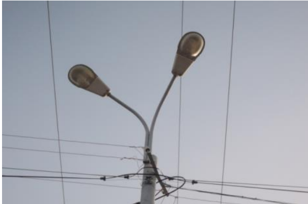
Picture 34: Old luminaries with 250W HPS lamps
