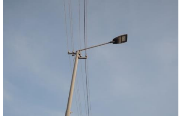
Picture 35: New 75W LED street lights
