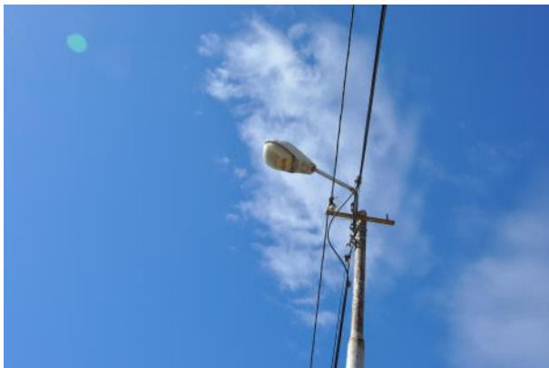
Picture 27: Old luminaries with 250W HPS lamps
